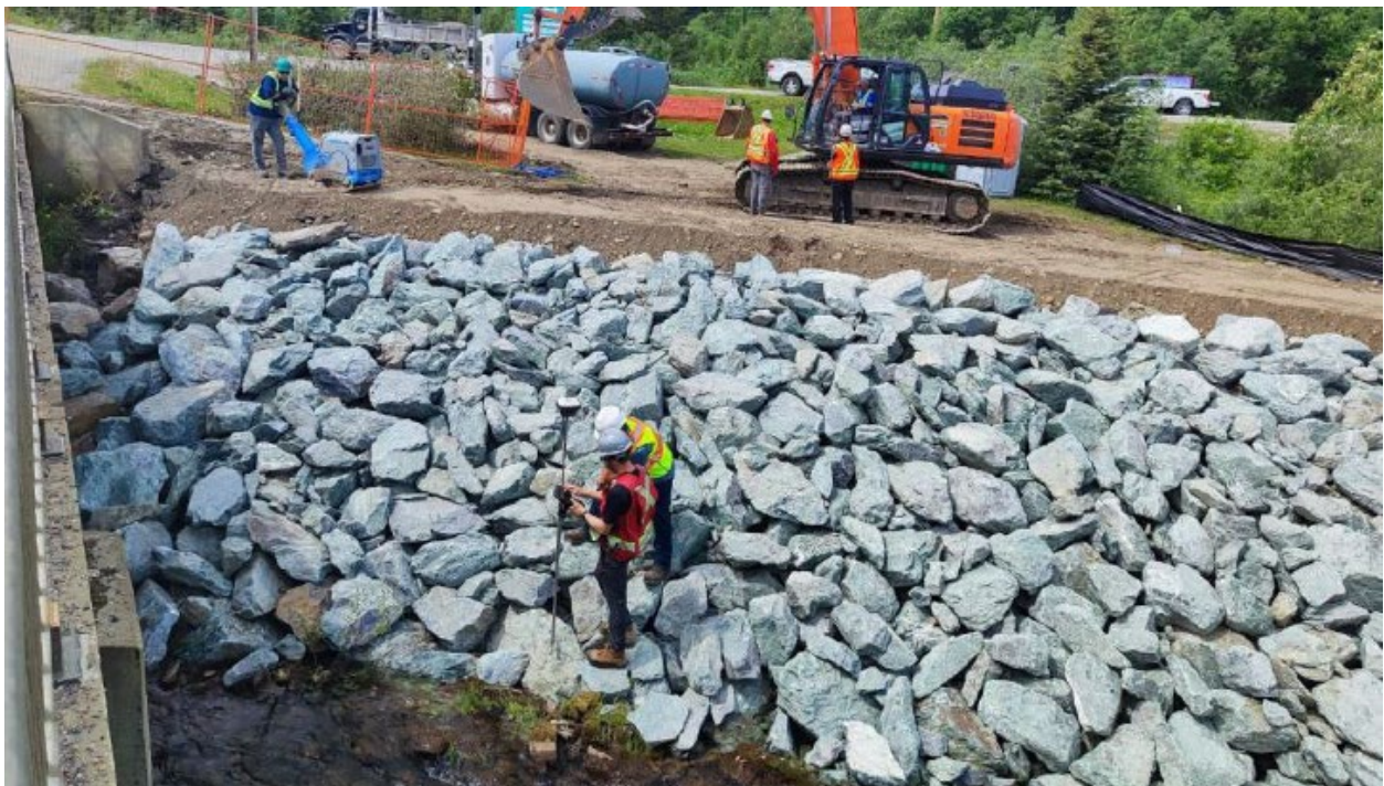
Figure 4-20 Riprap placement on the left (west) bank of Willow River immediately downstream of the Highway 26 bridge. Photo source: Radloff (unknown date).
