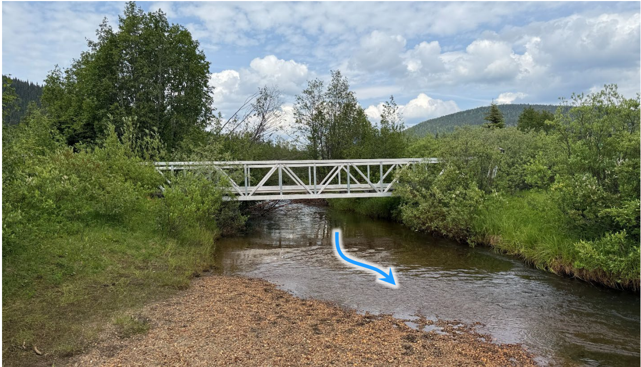
Figure 4-22 Upstream view of pedestrian bridge crossing of Williams Creek. BGC photograph of June 24, 2025.
