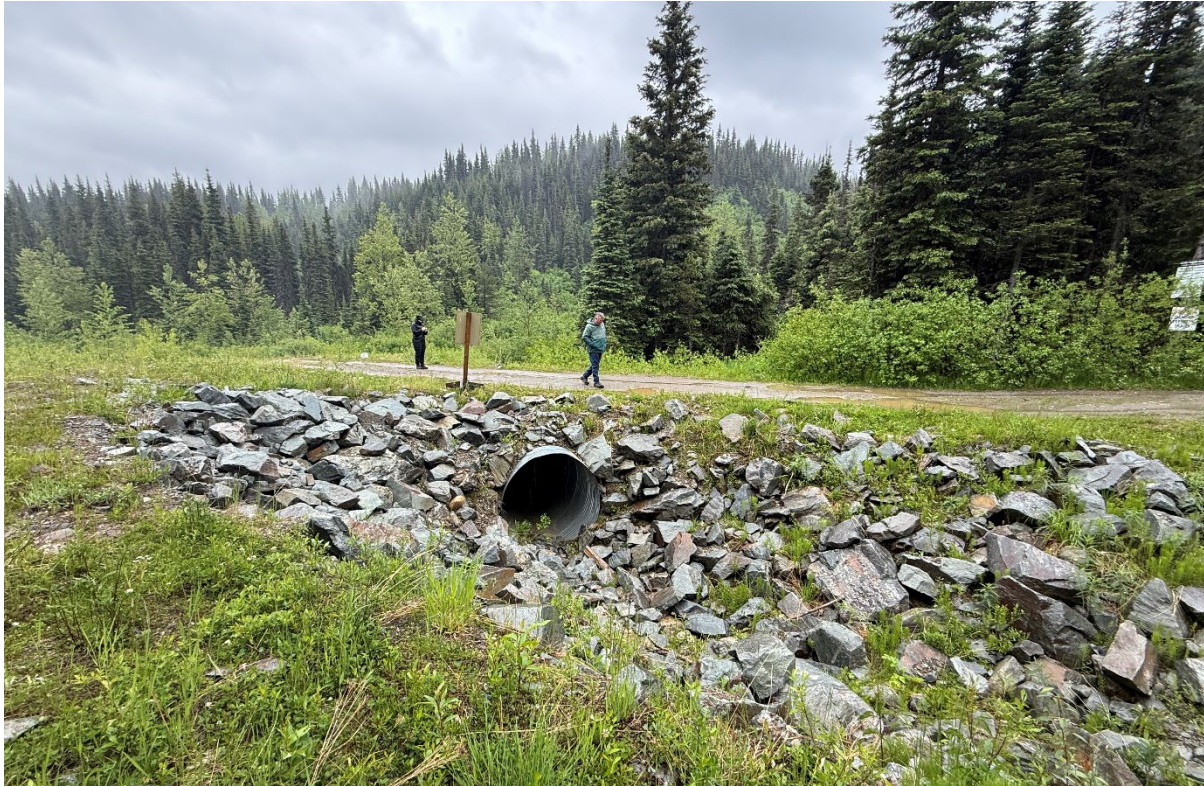
Figure 4-9 Downstream view of Stouts Gulch overflow culvert crossing of Richfield Road. BGC photograph of June 23, 2025.
