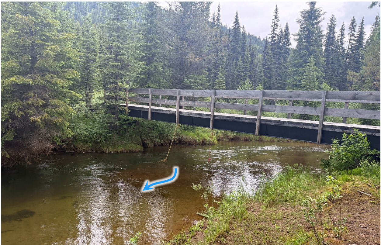
Figure 4-23 Upstream view of pedestrian bridge crossing of Willow River. BGC photograph of June 24, 2025.
