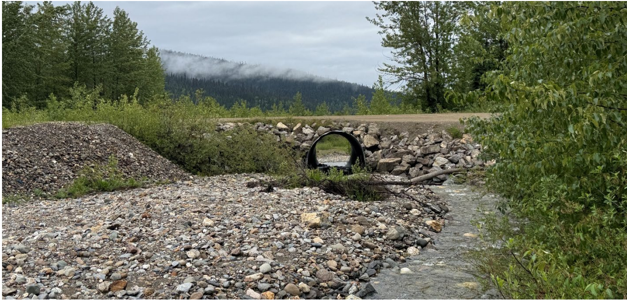
Figure 4-14 Downstream view of Williams Creek culvert crossing of Bowron Lake Road. BGC photograph of June 24, 2025.
