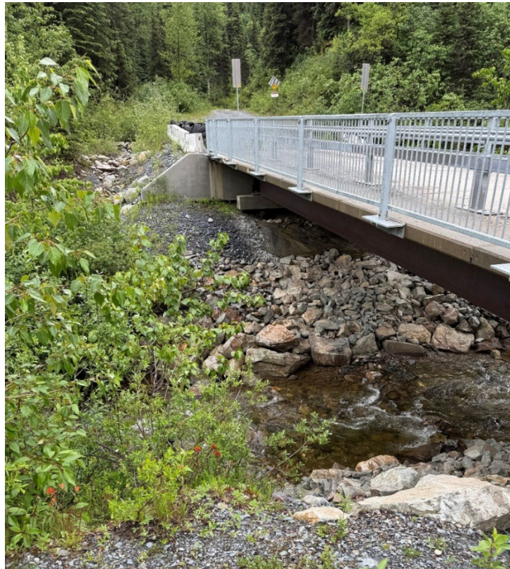
Figure 4-11 Upstream view of Prosperpine Bridge crossing of Williams Creek at entrance to historic Barkerville Town. BGC photograph of June 24, 2025.
