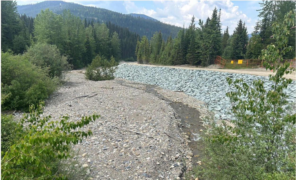
Figure 4-25 Downstream view of Lowhee Creek from the BGM bridge. The Phase 1 and 2a dike is visible on the right bank. BGC photograph of June 22, 2025.
